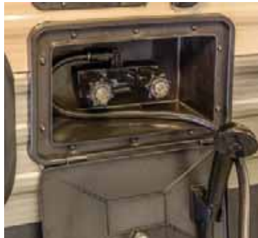
Outside Shower with Hot and Cold Water
