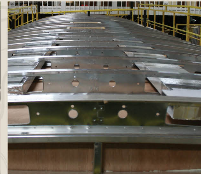
Walkable steel truss roof system
