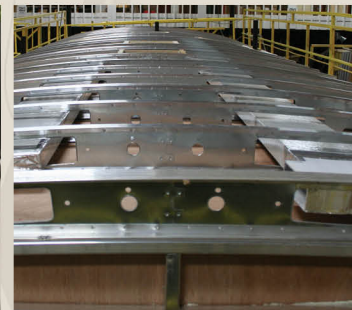
Walkable steel truss roof system
