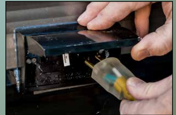
Convenient Outside GFCI Protected and Covered Outlet.
