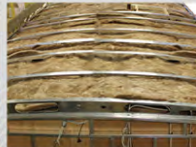
Aluminum truss roof system
